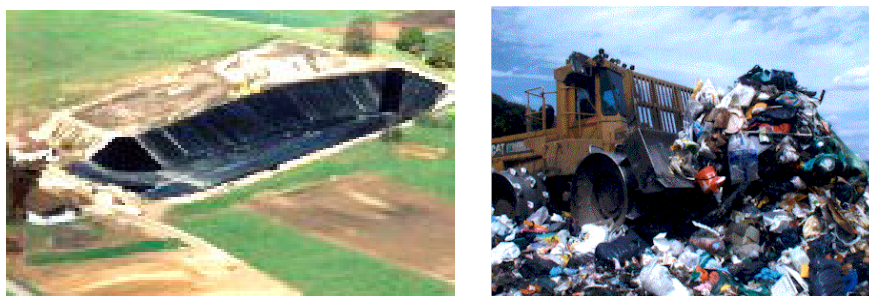
Fig. 5.1 A new and empty landfill site with visible bottom seal sheet (left) and waste placement and compaction in a sanitary landfill with special loader (right)
