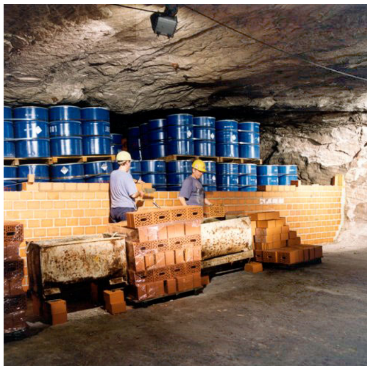
Fig. 5.5 Separation of one completed compartment by a brick wall in the underground deposit Herfa-Neurode. At the ceiling the rock salt vein is visible 11
